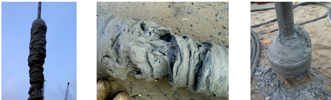
Figure 5. Failed grouting of the pile shaft.
